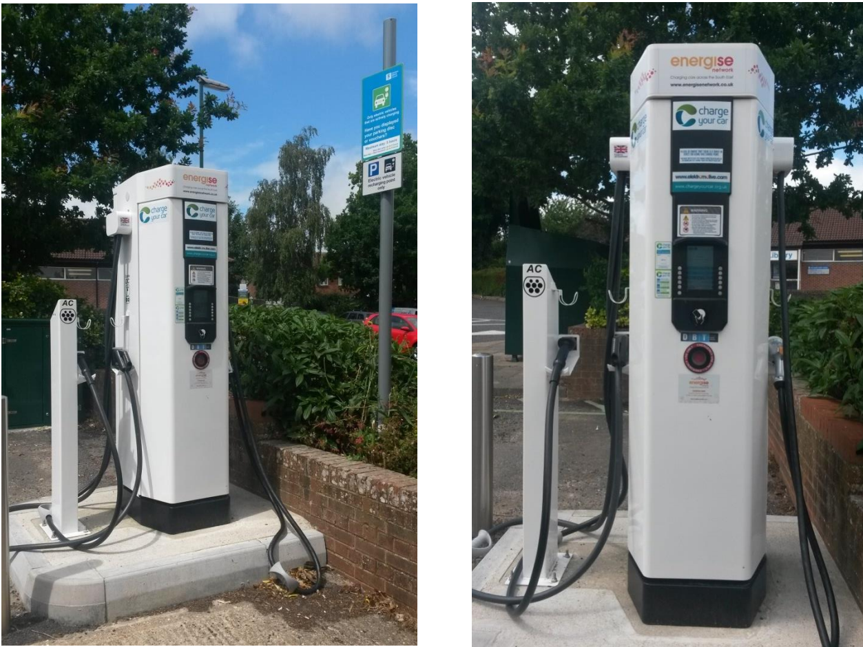
Figure 2.3 – Billingshurst eV Rapid Charging Point (Six Bells Car Park)
